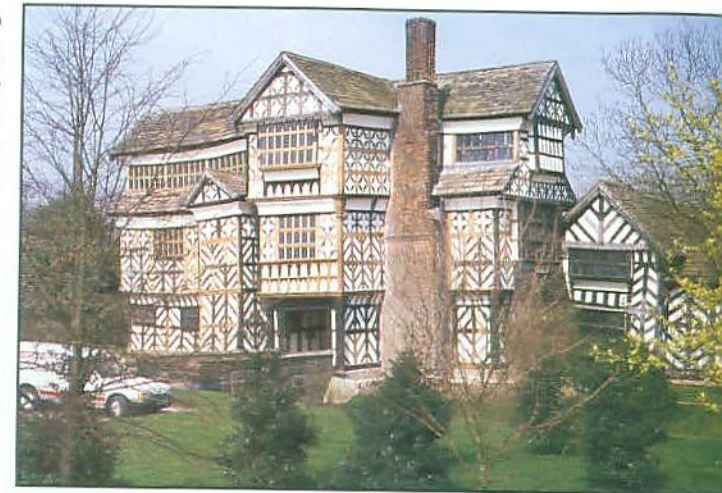
The South Range after repair. There are no plans to reblacken the timber (photo: The National Trust)
