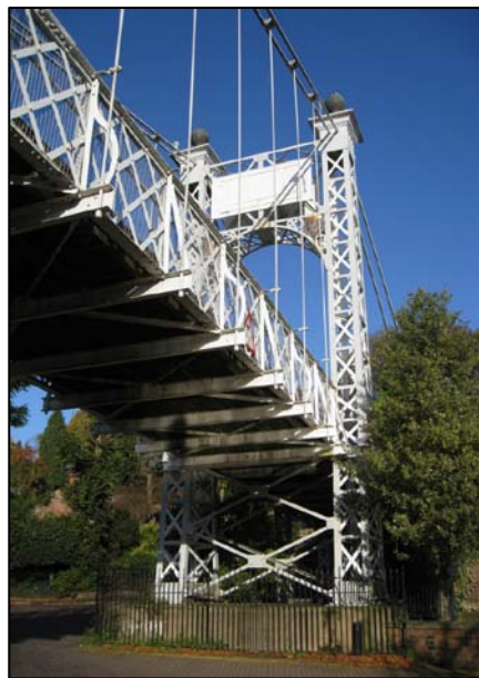
Figure 9: Bridge over the Dee at Queen's Park suburb. This bridge represents an important heritage asset contributing to the sense of place and character of suburban settlement (Cheshire HER)
